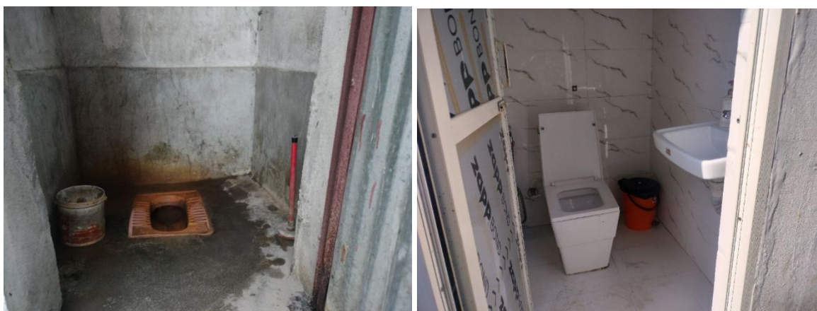
Figure 3: Sanitation technologies at households of Chandragiri Municipality.
