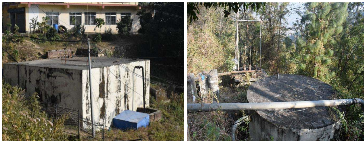
Figure 12: Reservoir tank of Dhankuta Municipality WSUC.
