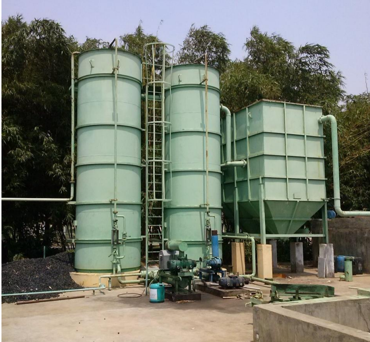
Mechanical STP Was giving trouble
