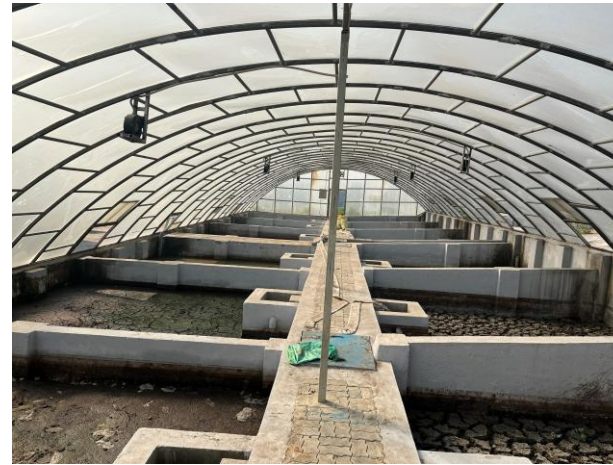
Sludge drying beds with GHSD, Angul FSTP
