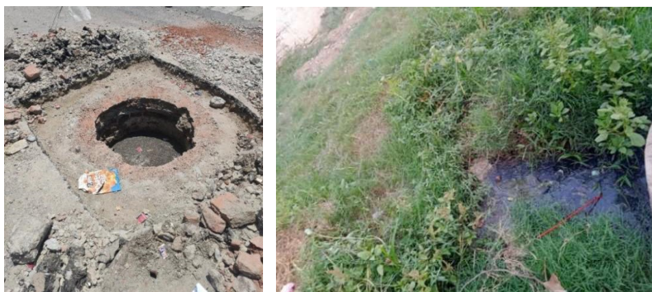
Figure 5: Offsite sanitation systems (Manhole of sewer network on left and discharge of sludge to an open environment on right) in Ratnanagar Municipality.
