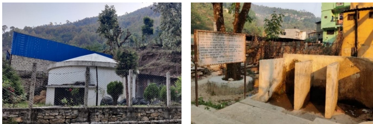
Figure 14: Reservoir tank of Tamghas Water Supply Scheme and Community tap at Resunga Municipality.
