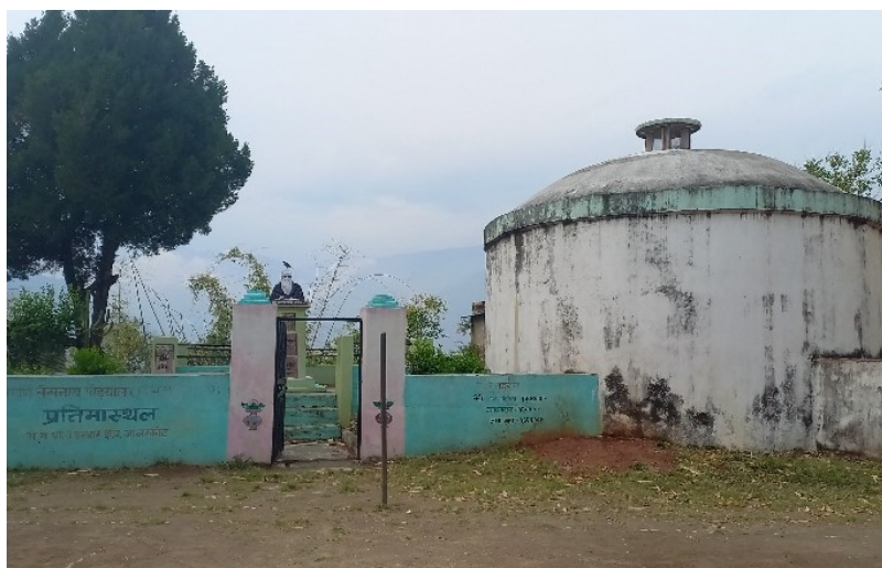
Figure 9: Reservoir tank existing at the Khalanga Bazar.
