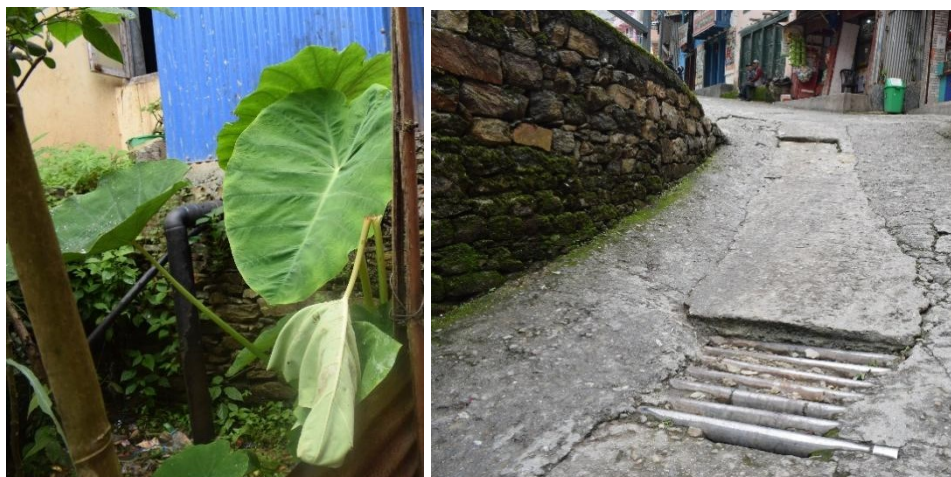
Figure 5: Toilet connection to a sewer network and sewer line in Siddhicharan Municipality.
