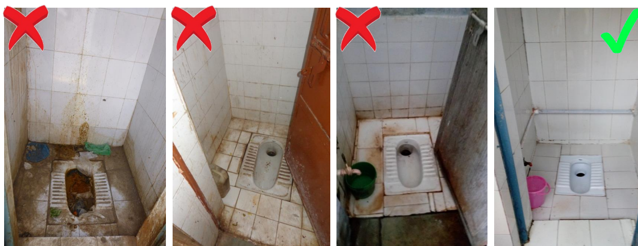
Figure 18. Cleanliness of a Toilet
