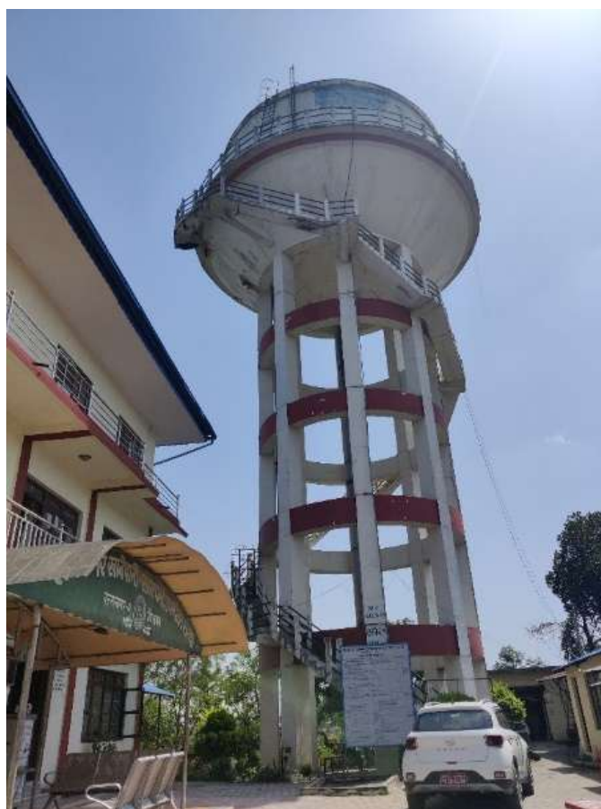
Figure 19: Reservoir tank for drinking water of Ratnanagar WSUC.
