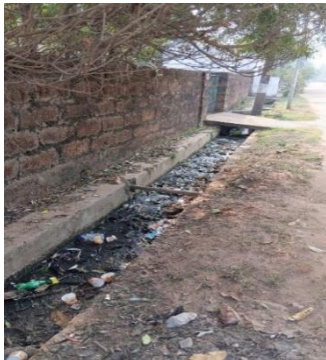
Figure 1: a. uncleaned open drain; b. closed drain overflowing on the street due to blockages, c. open drainage to agricultural field (Source: Chinmayee, Bulton, CFAR. 2025).
