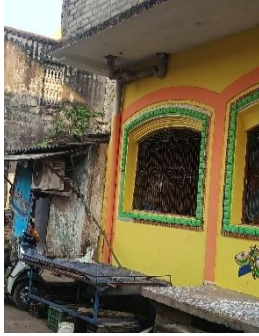
Figure 2: Toilet outlet directly connected to an open rain, and drain water discharged into open grounds (Source: Soumyashree & Bulton, CFAR. 2025).
