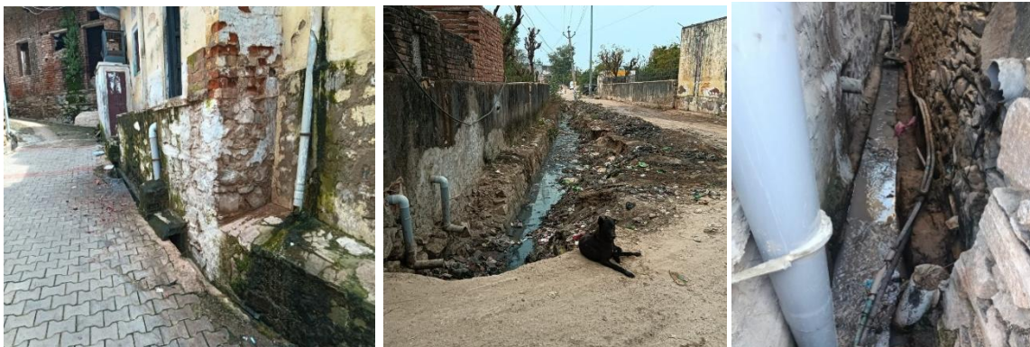
Figure 1: Toilets are connected to open drains (Source: Rajat, Asha, Suman. CFAR. 2025).
