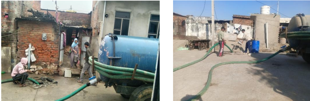
Figure 6: Containments are being emptied by cesspool operators. (Source: Sajna & Mamta, CFAR. 2025).
