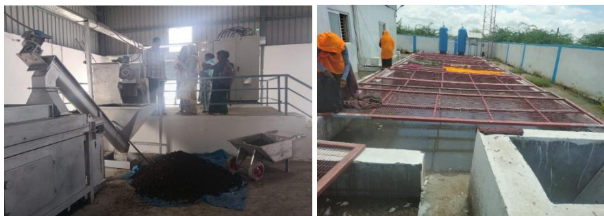
Figure 8: Sludge treatment operation in the FSTP. (Source: Madhu, CFAR. 2025).
