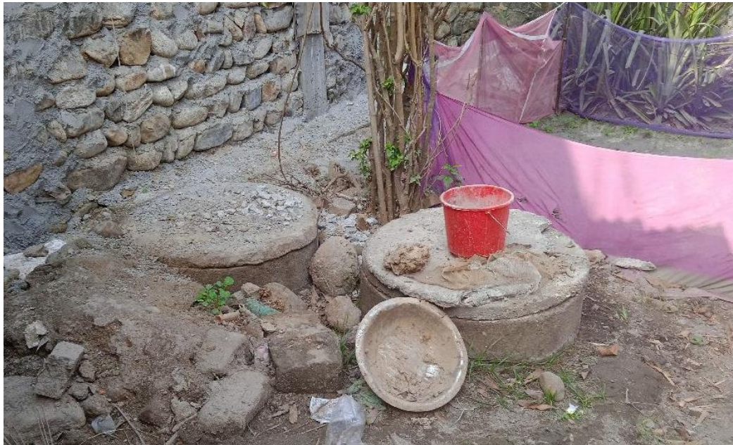
Figure 5: Inappropriate design of the twin pits, where the distance between two pits is less than 1 m.
