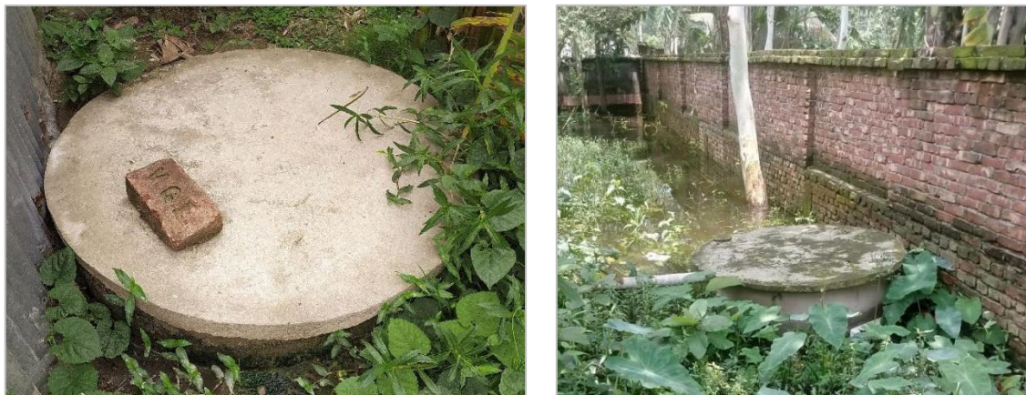
Figure 6: Containment technologies and their connections in Hakimpur Municipality. (Source: Field Survey 2023/ O.CREEDS_WaterAid Bangladesh).
