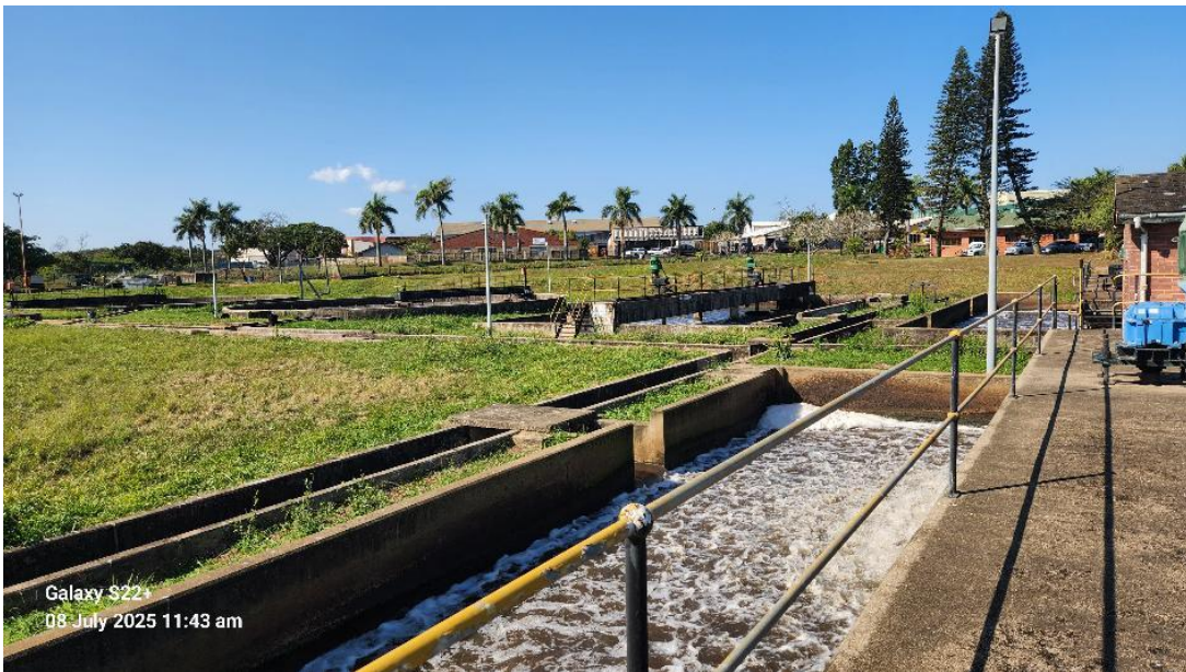
Figure 4: The Empangeni WWTW (a conventional activated sludge (CAS) plant).
