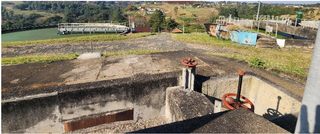
Figure 6: The Vulindlela WWTW.
