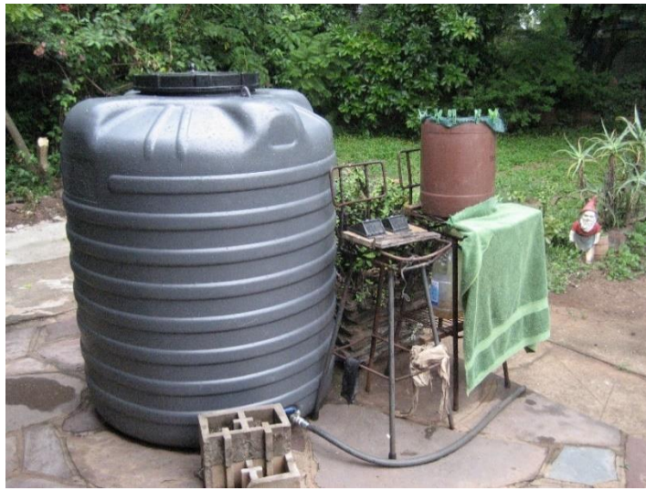
The outlet from the upper tank can be seen and links to a water pump to direct water to various tanks in the garden.
