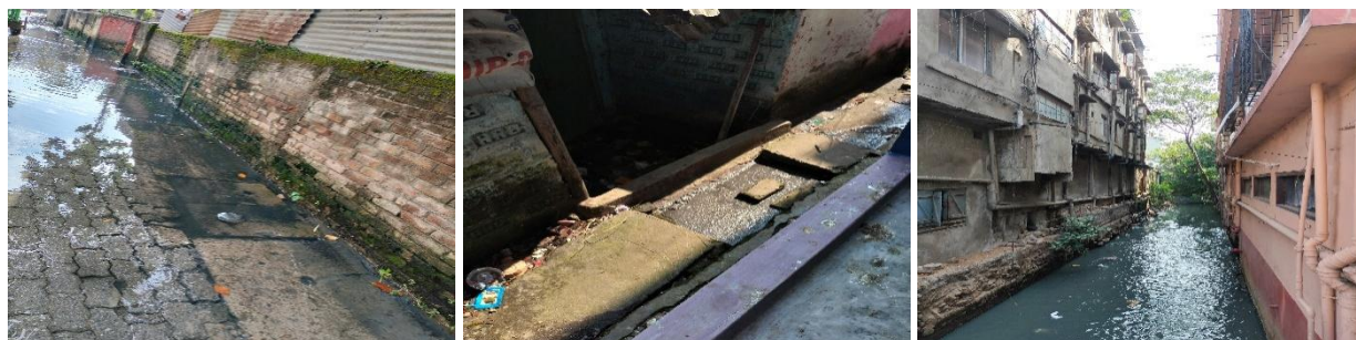
Figure 6: Overflowing Drain due to Water Pipe Leakage; Blocked Drain; Nullah/Drain (Source: Vikash/2024).
