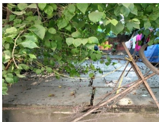
Figure 9: Septic Tank (Source: Vikash/2024).
