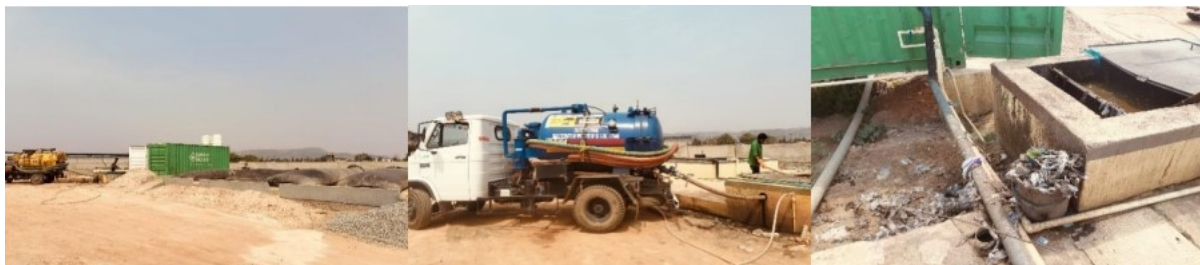
Figure 20: FSTP at Boragaon (Source: Vikash/2025).
