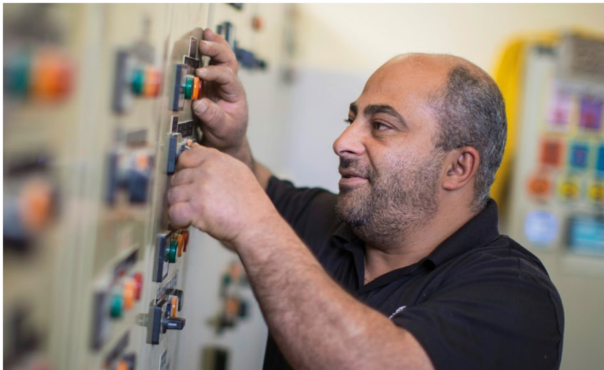
← Operator at the Fuheis wastewater treatment plant
