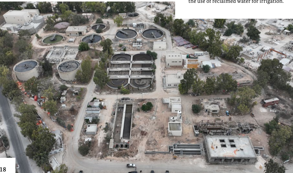
← Central Irbid wastewater treatment plant
