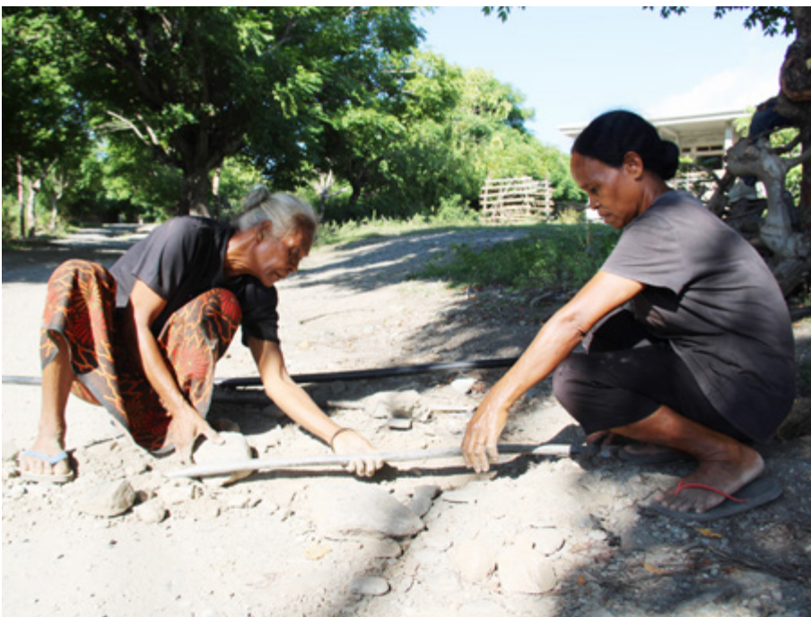
Women undertake operation and maintenance works on a piped water system in Liquiçã, Timor-Leste Credit: WaterAid Timor-Leste
