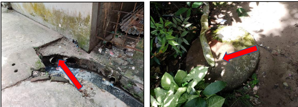
Figure 4: Left: Septic tank connected to a nearby drain. Right: Septic tank connected to soak pit (Source: Field Visit, 14 July 2021)
