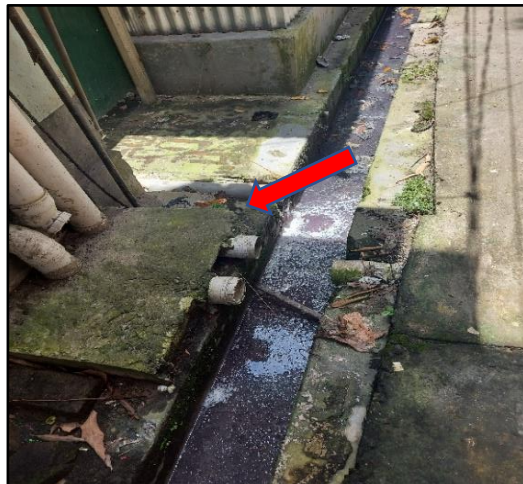
Right: Outlet connected to an uncovered drain
