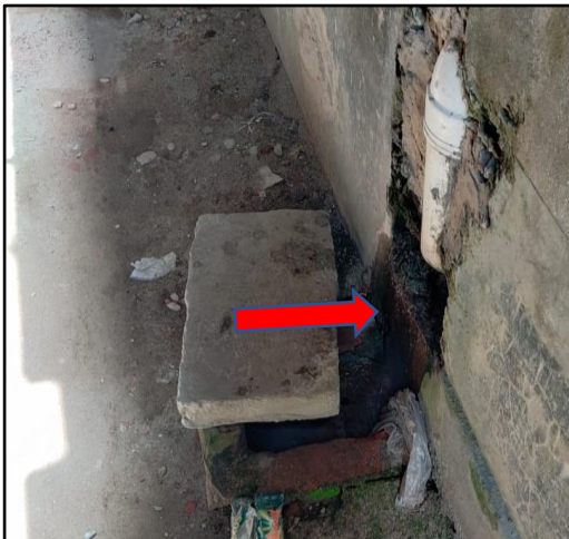
Left: Outlet connected to an uncovered drain
