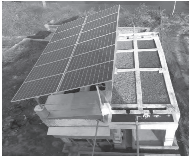
Top view on HRF/SSF/ACF filters with PV cover
