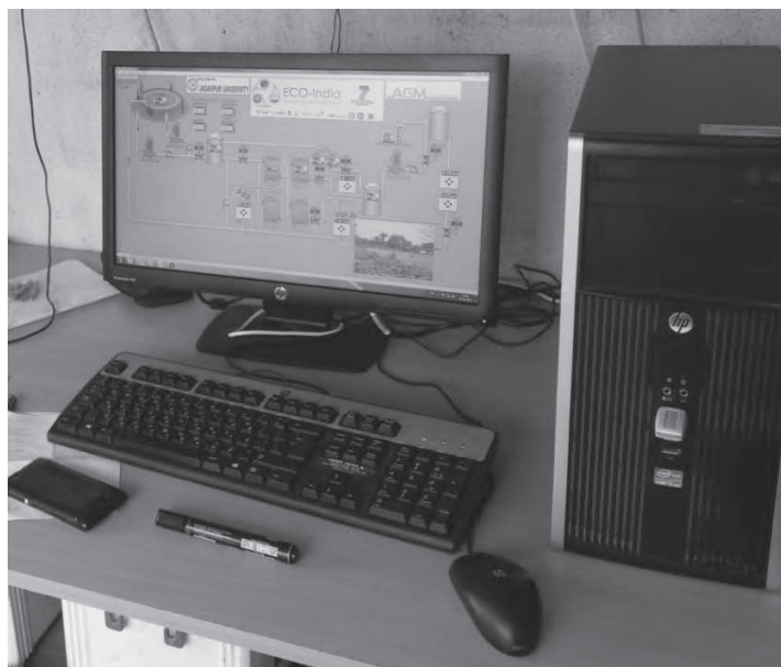
SCAD System for online monitoring
