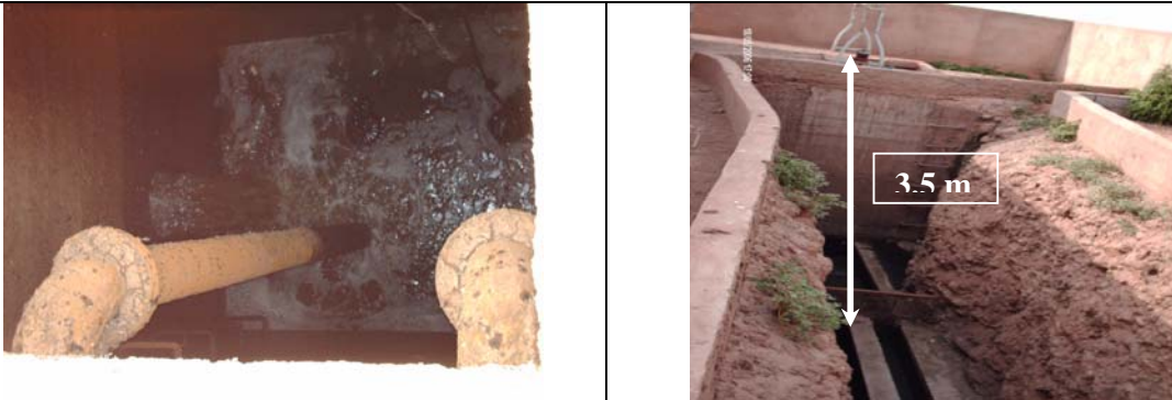
Figure 26: Station de pompage
