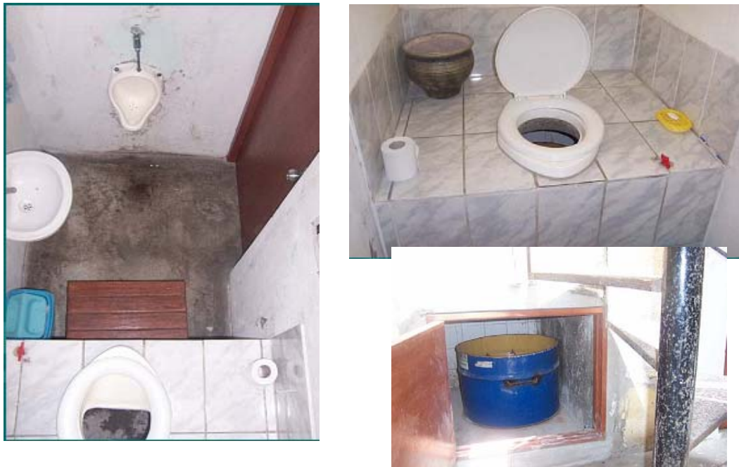
Figure 3-16: Ecological dry bathroom built inside the house in Lima by CENCA (Luna, 2005)
