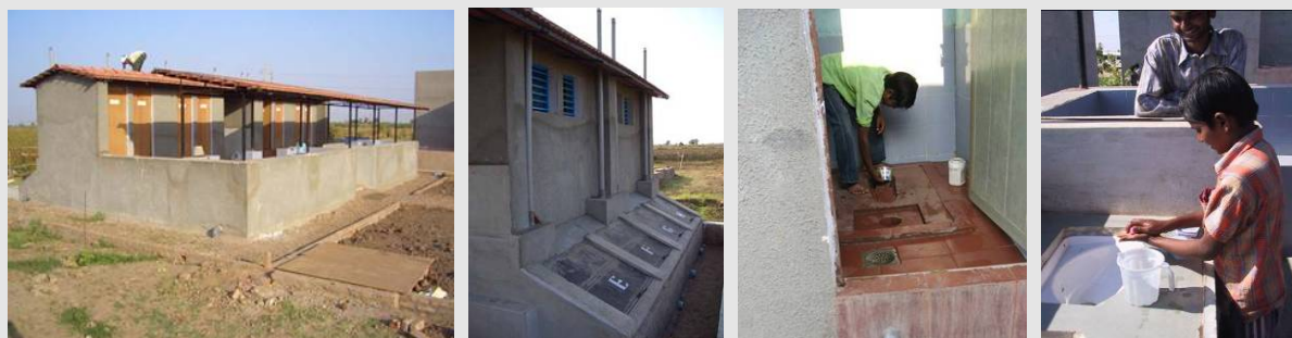
Figure 7: The school's sanitation block (far left), and from the back (left). Faeces are not flushed with water, but sprinkled with dry material, e.g. ash, over them (right). Hygiene education, such as hand washing is part of the scheme (middle). (Source GTZ/ESF)
