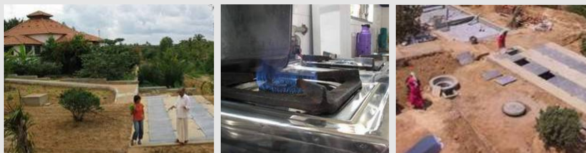
Figure 11: Surroundings of Camphill Trust building do allow reuse of treated water and produced fertiliser (left) Biogas is used for cooking (R) Biogas plant with sludge drying beds (L) (Source BORDA)
