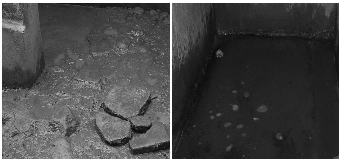
Photograph 1. Toilet floors wet with urine in one of the schools
