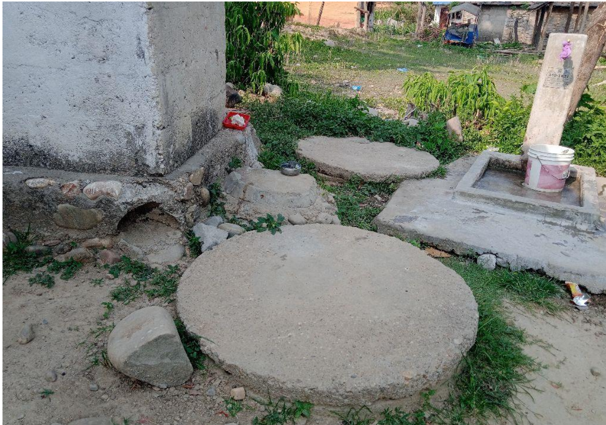
Figure 5: Twin pit installed in the household at Kamalamai Municipality.
