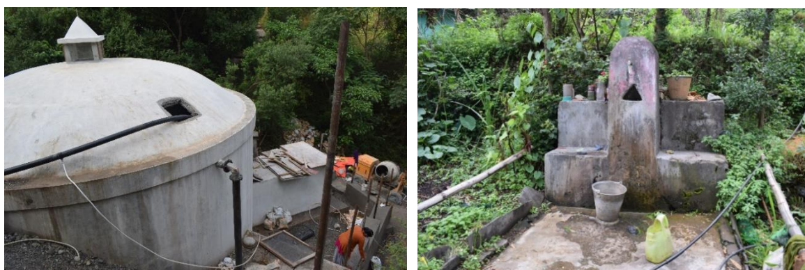
Figure 13: Water intake and piped drinking water supply.
