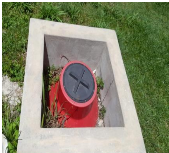
Figure 10: Precast plastic ST (Source: Jodian/Org./2022).
