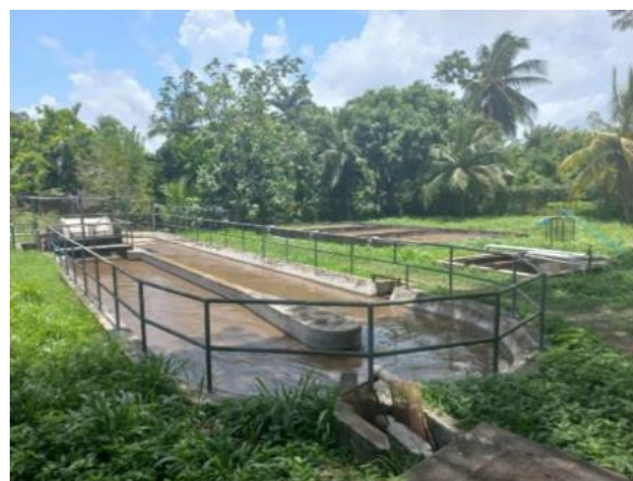
Figure 4: STP, operated by NWC (Source: Jodian/Org./2022)
