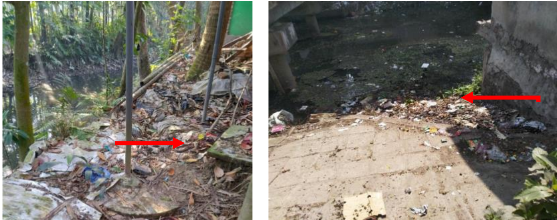
Figure 6: Containment technologies and their connections in Magura. Left: Septic tank connected to the nearby water body. Right: Toilet pipe connected to open drain. (Source: Feasibility study 2020-21/DPHE).
