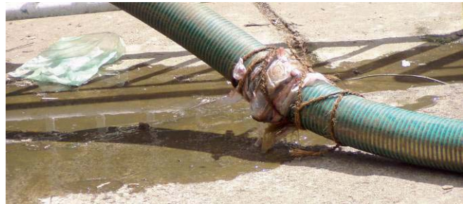
Improper fittings and hose connections cause leaks that must be disinfected with bleach or lime after pumping. Always leave the site clean after pumping.
