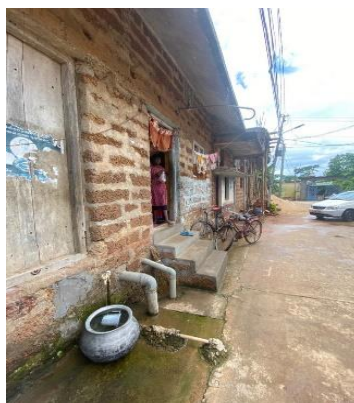
Figure 7: Septic tank connected to open drain, Ward 3 (Source: Dimple Behal/CSE).
