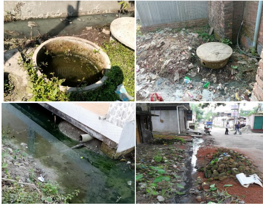
Figure 5: Open as well as covered ring pits and outlet of the septic tank connected to open drain (Source: Field Observation, UIIPF/DPHE, 2020).
