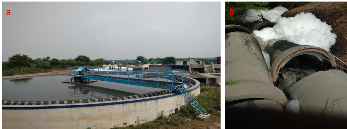
Figure 1.18: A) Aerobic Treatment Plant Unit at Thanjavur, b) Treated Effluent Foaming at the Outlet Point
