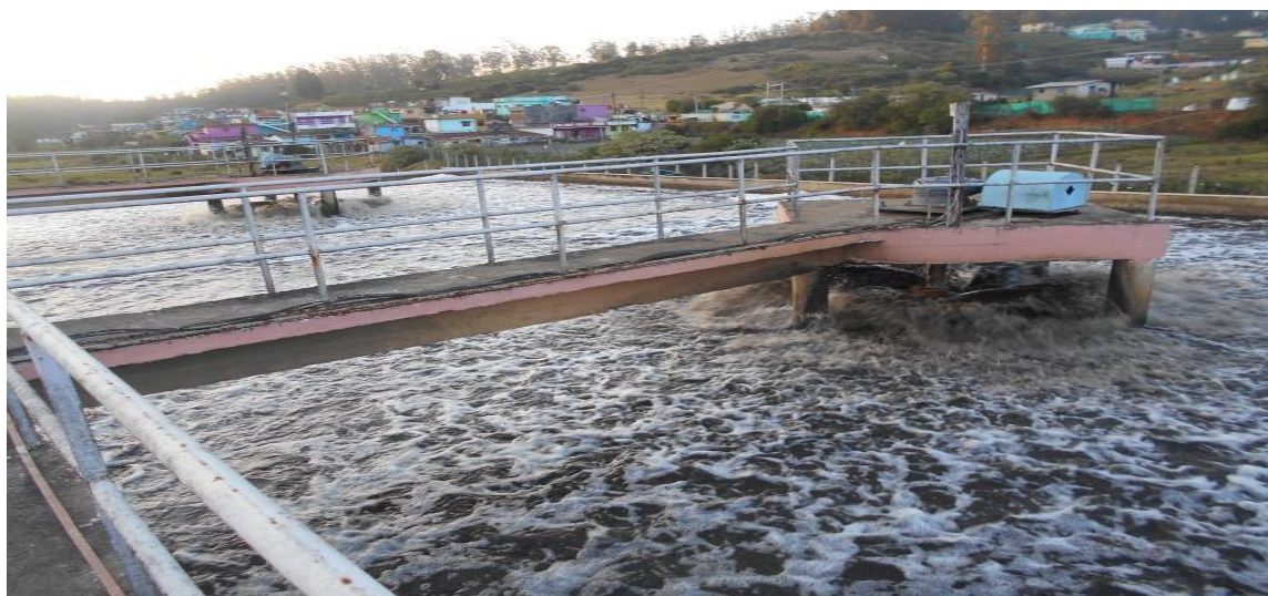
Figure 1.19: Aeration Treatment Module at Ooty
