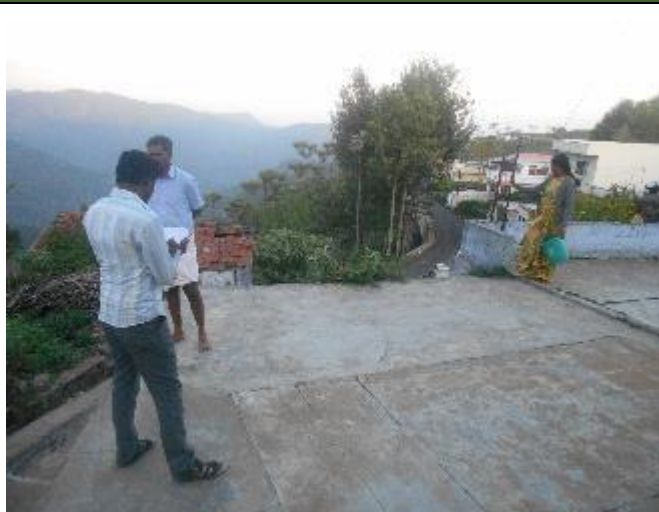
Figure A5.1: Septic Tank Constructed in a Hilly Zone of Tamil Nadu
