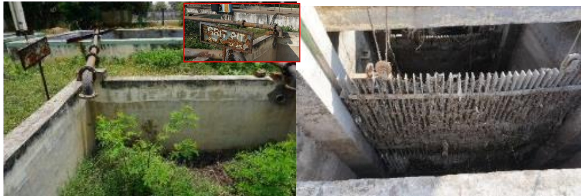
Figure 3.1: Grit Pit and Screening Systems – Not Being Maintained in Anna Stadium
