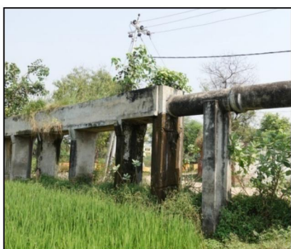
Mixing tank of sewage and tubewell water
