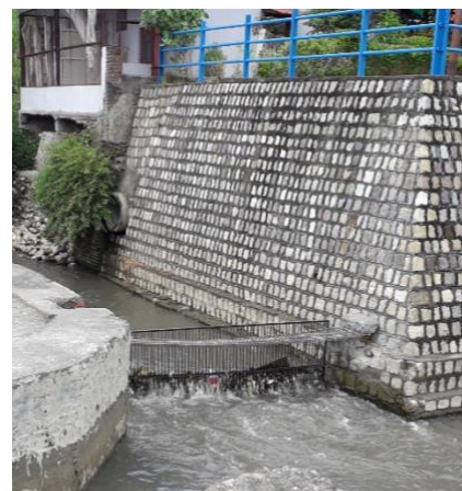
Figure 3: Bar screens installed at Chandreshwar Nala for intercepting solid waste (Rahul/GIZ, 2018)
