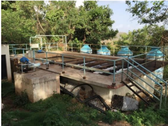
Photo 1: Sewage treatment plant
