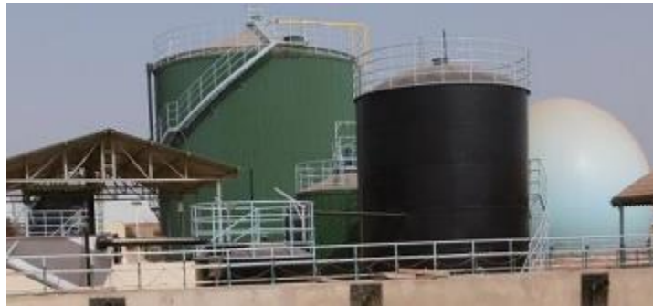
Figure 11: Biogas and electricity production unit in Ouagadougou (SNGFAEUE, 2017)
