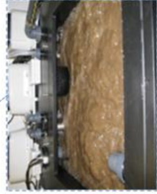
5 - Membrane bioreactor (MBR) Volume of tank 480 l
