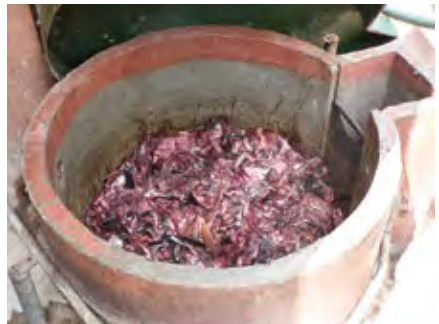
Picture A4: Inlet of Sreekaryiam biogas plant (photo: Sandec).
