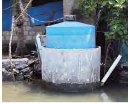
Picture 33: Biogas plant discharging directly into surface water (photo: Sandec).
