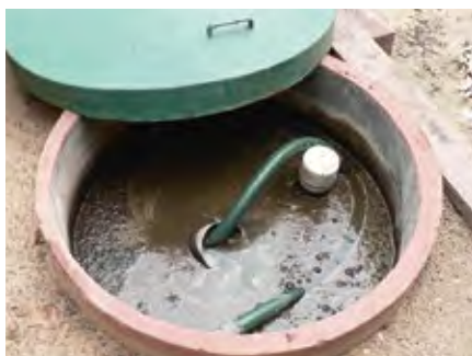
Picture A7: Effluent tank at the Sreekaryian biogas plant (photo: Sandec).
