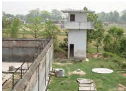
Picture E1: Biogas sanitation system in Nepali prison with solid waste feeding chamber, gas outlet, underground dome and effluent pit outside the prison wall (photo: Sandec).
