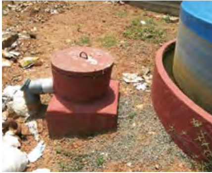
Picture 32: Outlet that is directly connected to sewer system (photo: Sandec).
