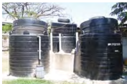
Picture D1: ARTI biogas plant at Azania Secondary School (photo: Sandec).
