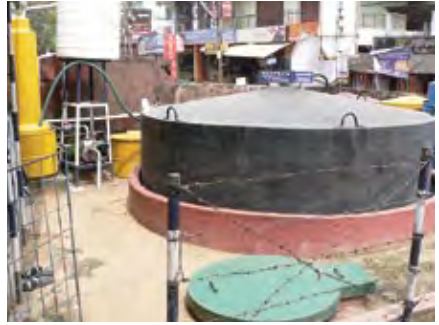
Picture A2: Floating drum biogas plant at Sreekaryiam fish market (photo: Sandec).
