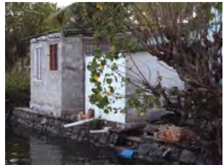
Picture B2: Toilet discharging into backwaters (photo: Sandec).
