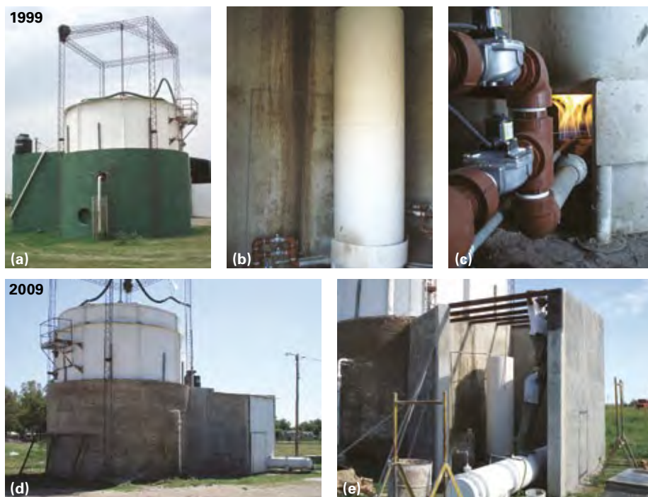
Picture G2: AD plant in Gobernador Crespo: a) before modernisation, b) water heater, c) automatic burner, d) after modernisation, e) protected components (photo: Eduardo S. Gropelli).
