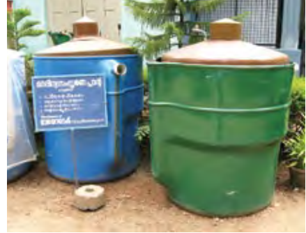
Picture 11: Above ground floating-drum digester for households in India, made of fibreglass reinforced plastic (photo: Sandec).
