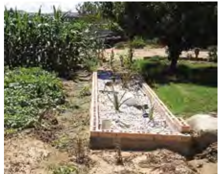
Picture 35: Newly constructed planted gravel filter with ABR (on the right). TED-BORDA, Lesotho (photo: Sandec).
