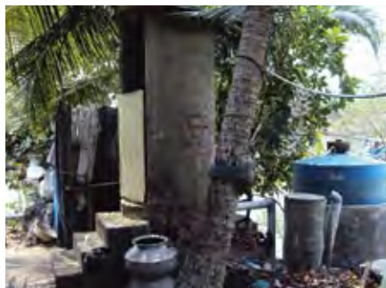
Picture B4: Toilet connected to biogas plant (photo: Sandec).
