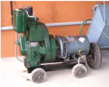
Picture 28: Biogas engine (5 kW) in Thiruvananthapuram, India. The electricity is used for public lighting of streets (photo: Sandec).
