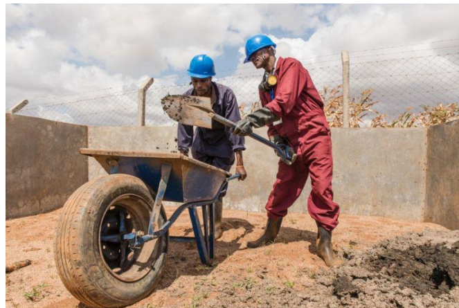
Photo. 6: Operators collecting the sludge in the drying beds at the DTF in Machakos © GIZ/Berea (2017)
