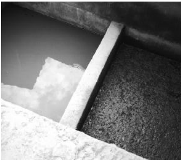
Fig. 9. Partition wall retaining scum. Inlet is at the right side, water flows below the partition wall into the compartment at the left side. [photo: Sasse]
