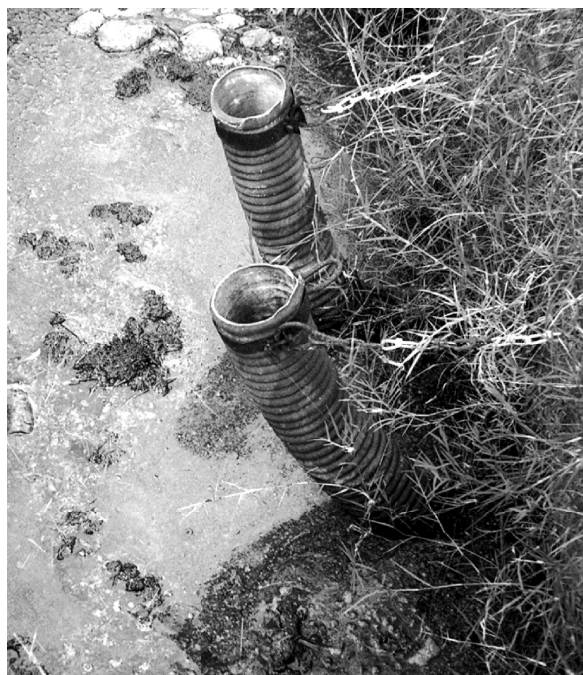
Fig. 54. Flexible pipes for de-sludging. Sludge is discharged by hydraulic pressure when lowering the pipe. [photo: Sasse]
