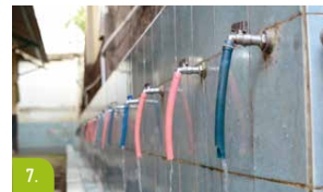
7. Make sure the water flows adequately to all outlets.
