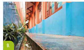
9. Ensure proper drainage.
