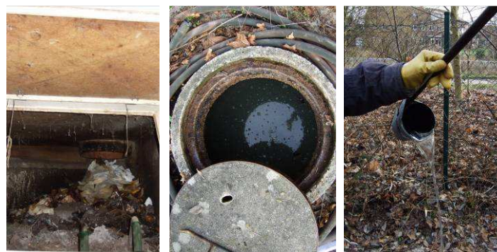
Fig. 10: Compost heap inside the composting container of the toilet (left), greywater in Imhoff tank (middle) and final effluent from constructed wetland (right). Source: A. Schöpe, 2009.
