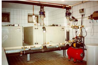
Bio-reactor for 6 apartments
