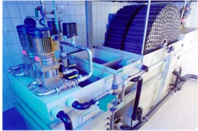
Rotating biological contactor for 24 apartments
