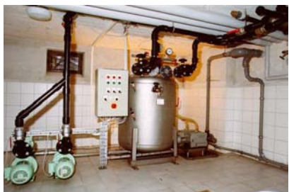
Vacuum pumping unit
