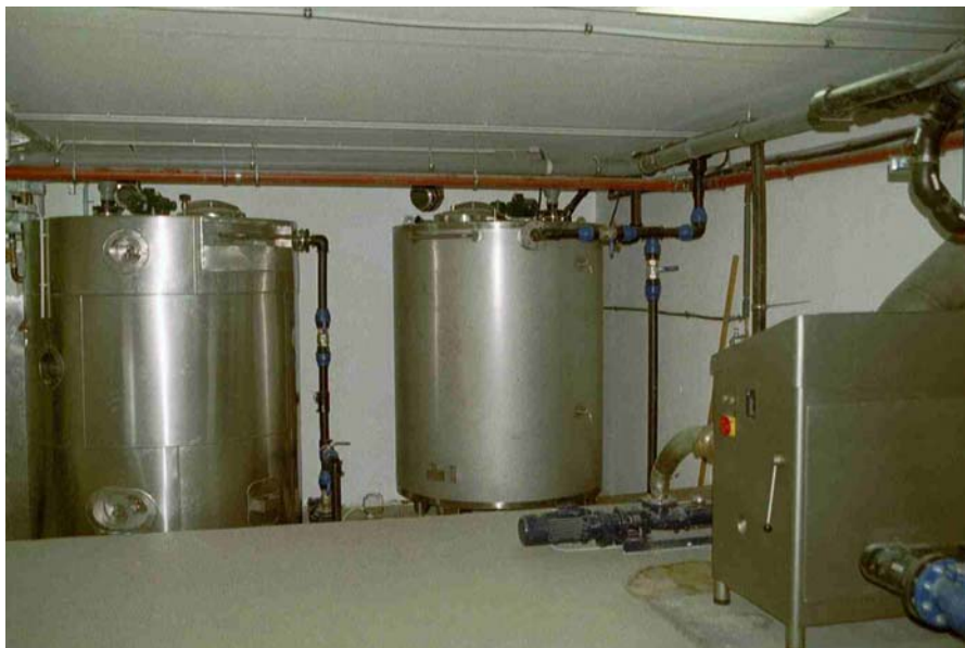
Figure 6: Mixing and hygienisation unit (source: Otterwasser) kitchen and bathroom) is transported by gravity pipes to several constructed
