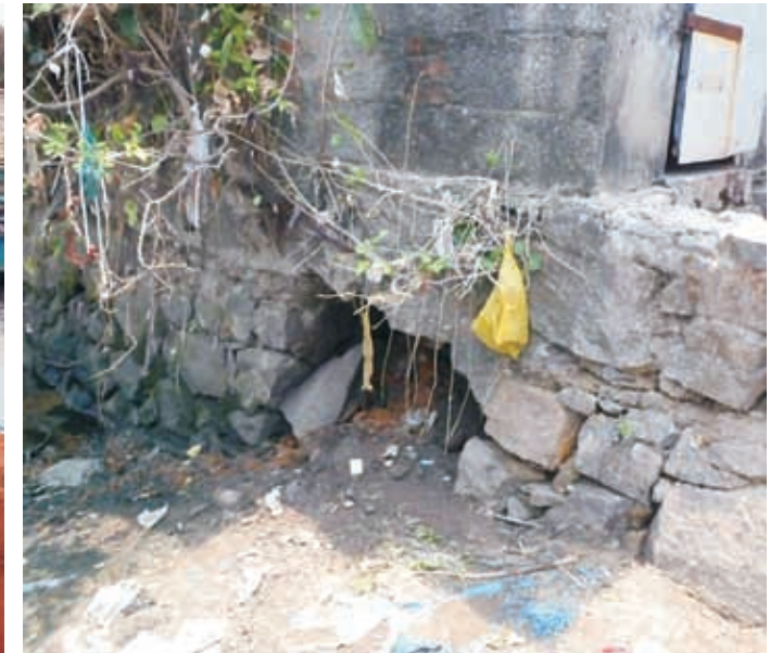
Figure 9: Inadequate septage management
