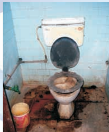
Figure 11(b): Poor condition of CTC
