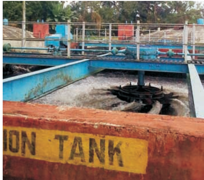
Figure 8: GCDMA's sewage treatment plant at Marine Drive
