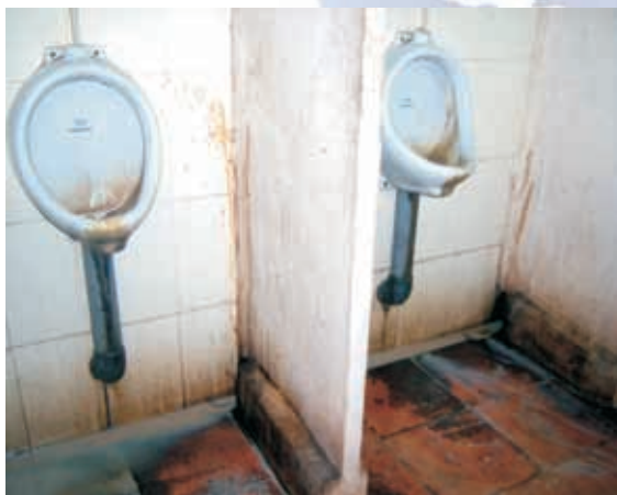
Figure 11(a): Poor condition of CTC
