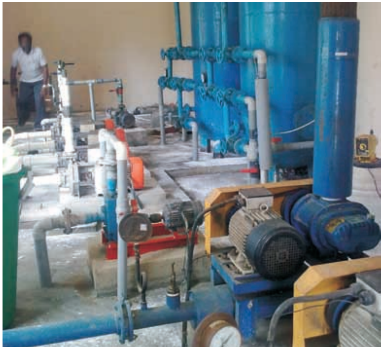
Figure 32: Hi-rise buildings-Inhouse Sewage Treatment facility
