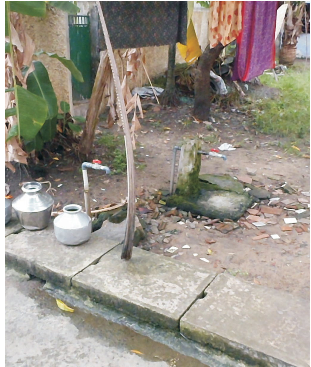
Figure 35: Poor service delivery of water supply
