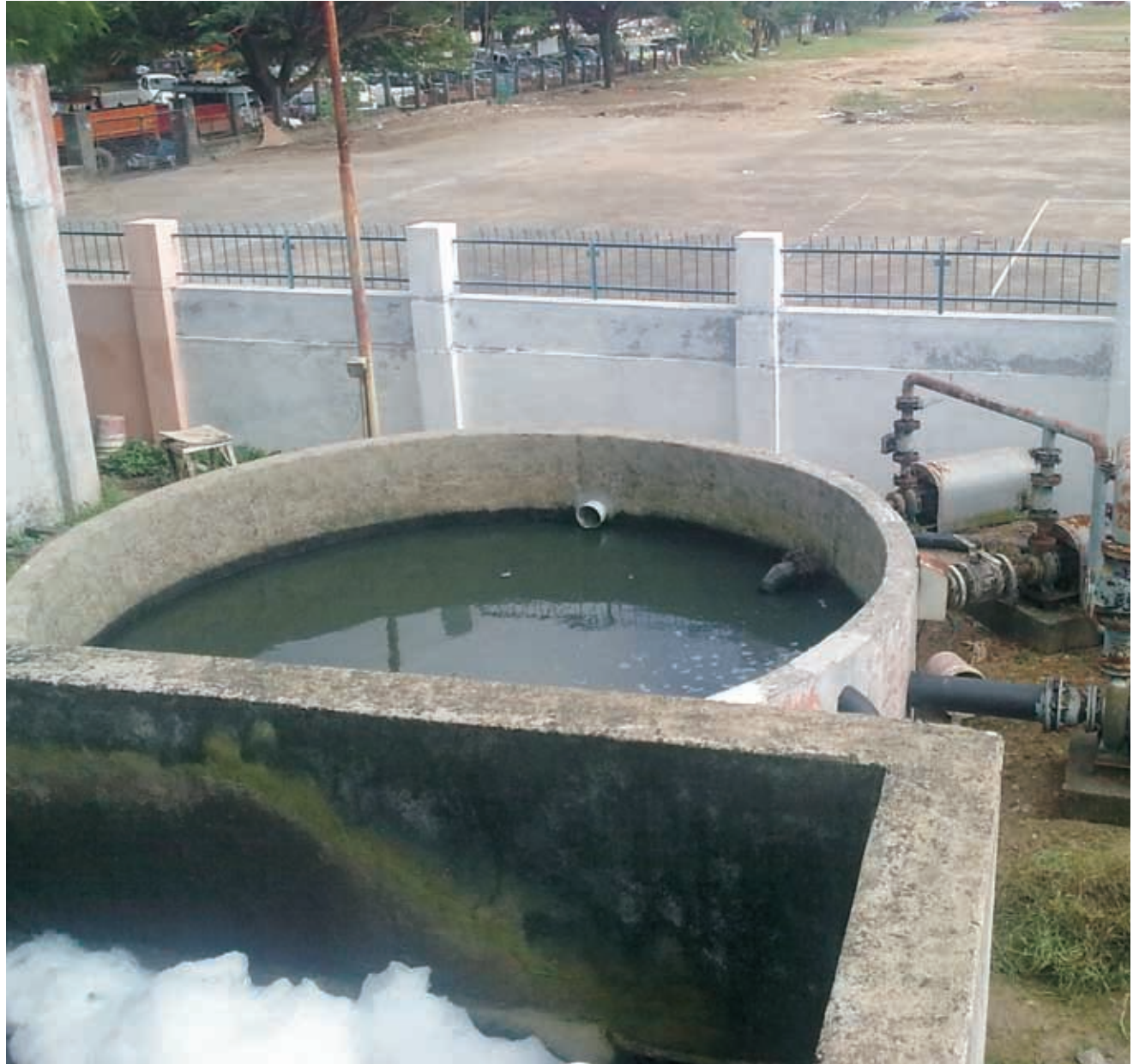
Figure 33: GCD A Sewage Treatment Plant at Marine Drive
