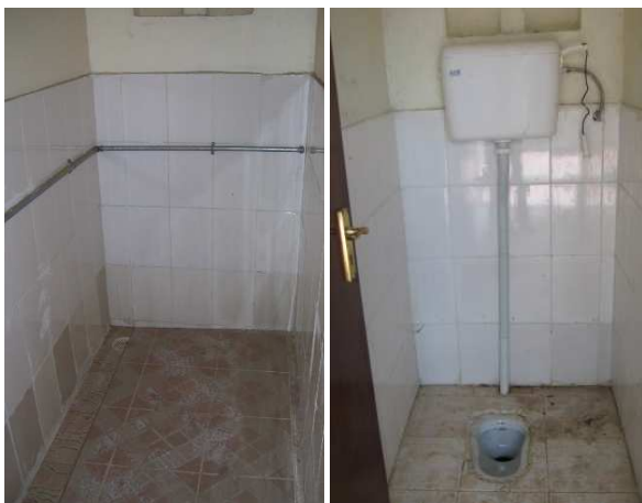
Fig. 6: Left: Urinal using a tiled wall (no door) with optional water flush. Right: Squatting pan with 10 L cistern (flush toilet); but these days a manual pour flush system is used for toilet flushing (see Fig.7).
