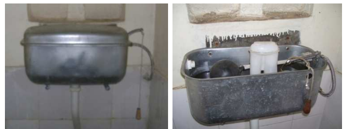
Fig. 13: Cistern after installation (left) and after vandalism/misuse and theft (right) a few weeks later. Repairs were undertaken by WSP, but the toilet operator now shifted to a pour flush system.
