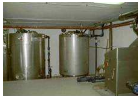
Fig. 9: Mixing and hygienisation unit, (source: Otterwasser)
