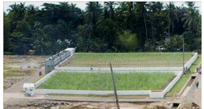
Fig. 8: Constructed wetland when construction was just completed in September 2006 (source: GEOPLAN Cebu). On the left side, the header tanks are visible.
